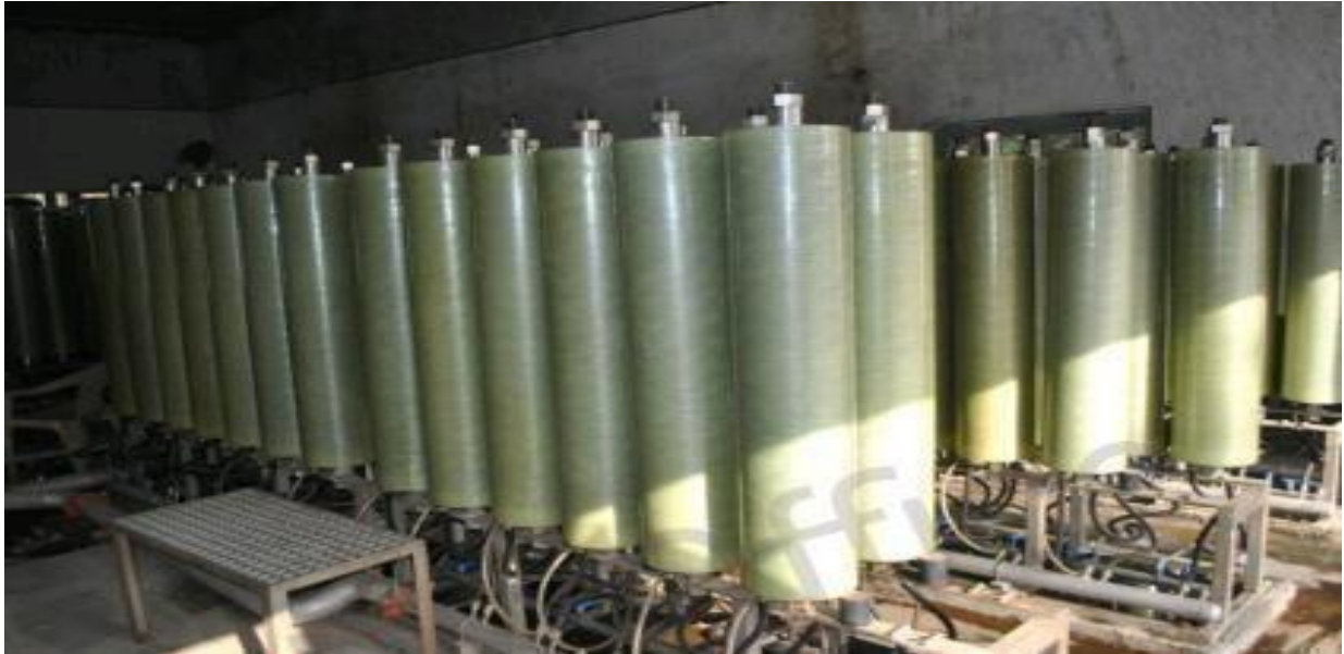
(PT RO PLANT)
